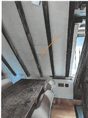
29. Staining below access panel in attic flat
