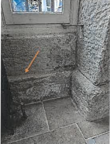
22. W window in Community Area- Salt efflorescence at low level and powdering on top of plinth
