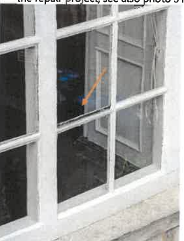
17. W side window with missing putty to glass
