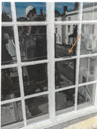
15. N window with missing putty to glass
