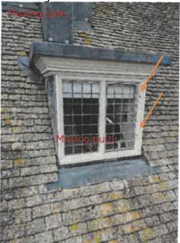
13. E side of the roof Pintols may be damaging frame
