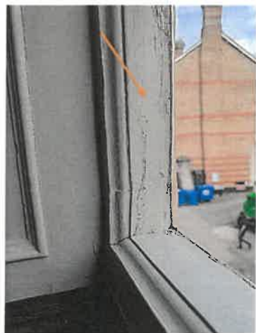
27. E window on first floor; possible water ingress through defective putty
