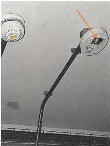
28. Missing cover to carbon monoxide sensor in boiler room
