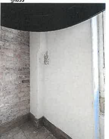
18. Damaged plaster W side below stair
