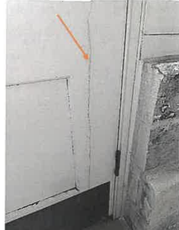
24. W door on S side; possible water ingress through gunstock joint.
