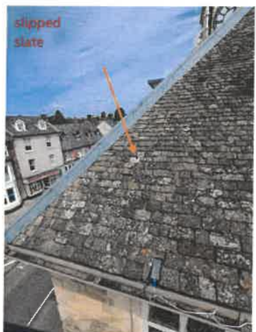
6. S slope- Missing slate temporarily replaced
