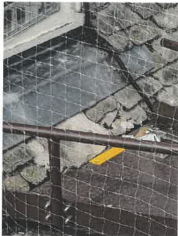
1. Damaged slates below the N dormer above flagpole gantry
