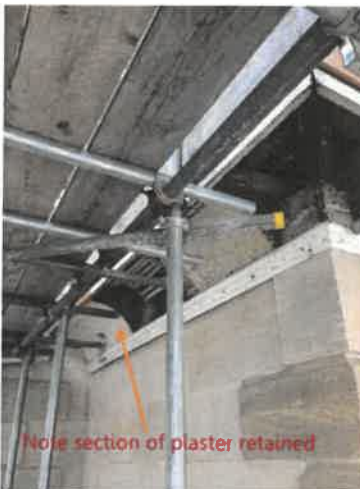
14. The W side of the N covering during the repair project; see also photo 31
