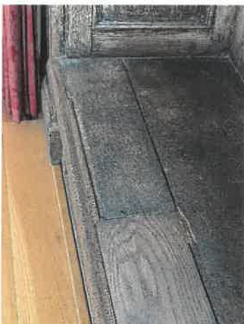
26. Damaged window seat on first floor E side.
